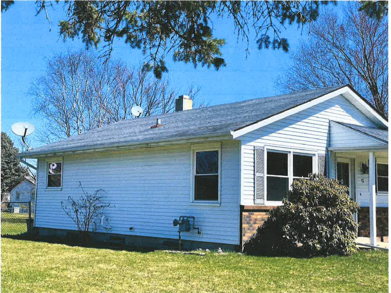
Side view from sidewalk. Worn and missing shingles, rusty vents.
