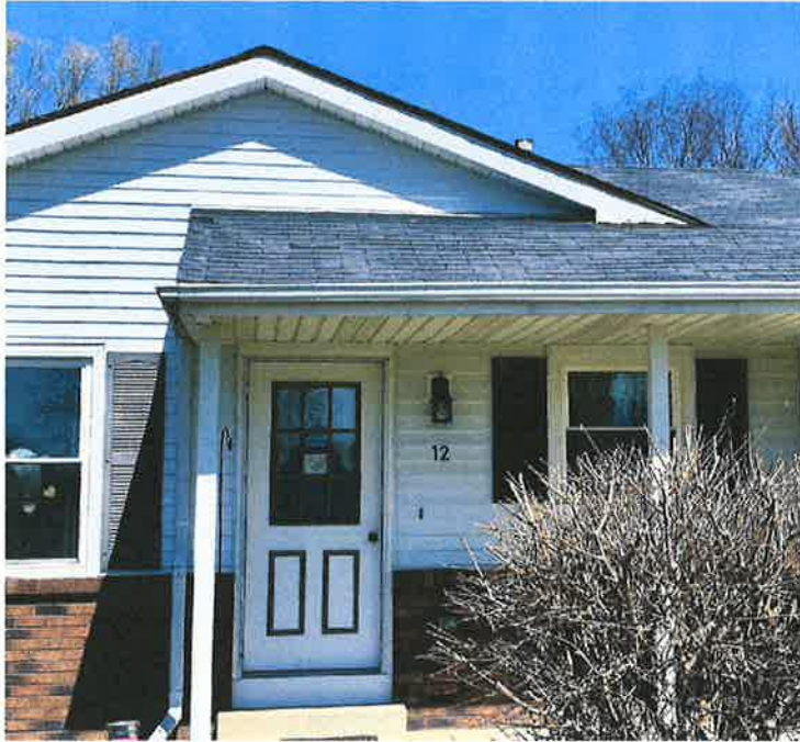
Sagging porch roof, missing and worn shingles. Missing storm door.
